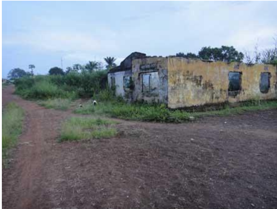
Goats and Sheep graze around the green vegetation of damaged houses left bare without windows, doors or roofing.
